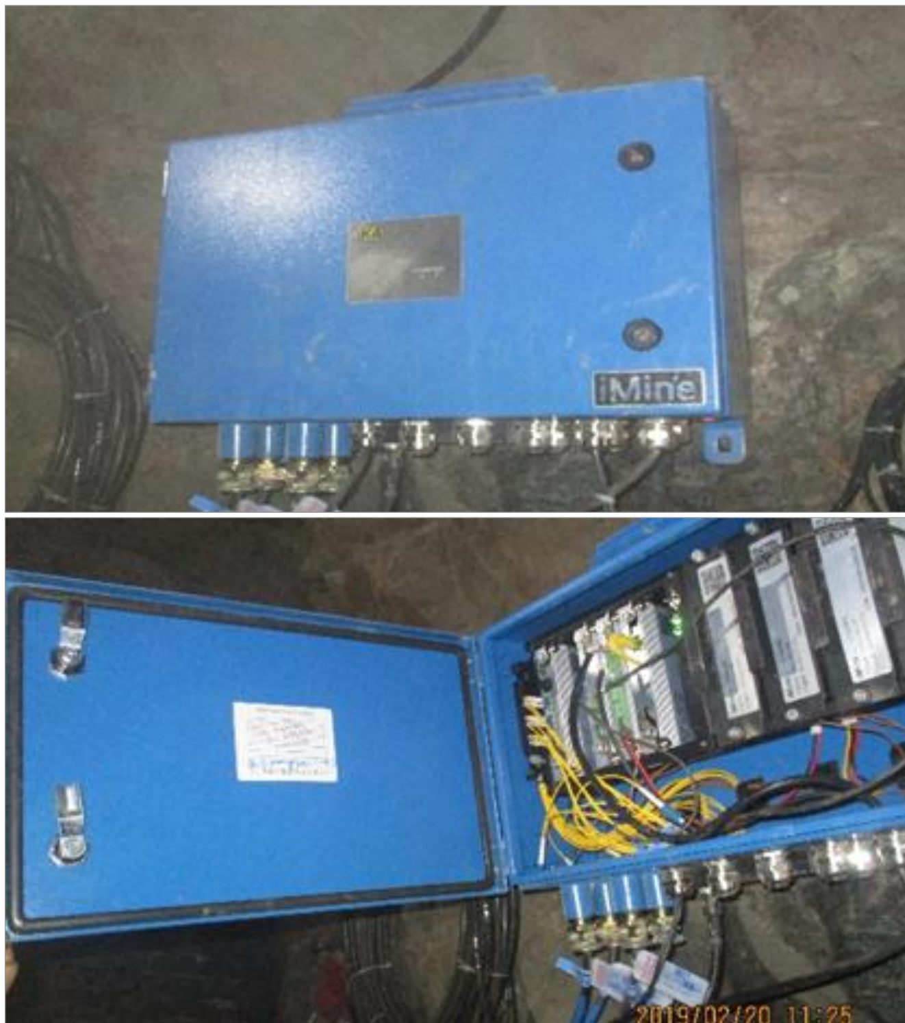
Figure 18.19 Modular base station at underground personnel positioning system
