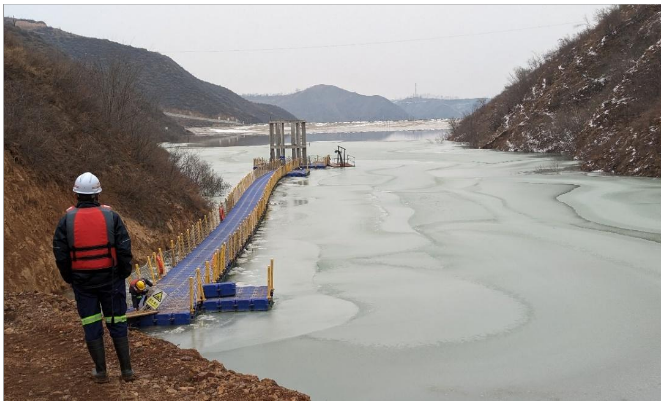
Figure 18.8 Operational decant tower in TSF2
