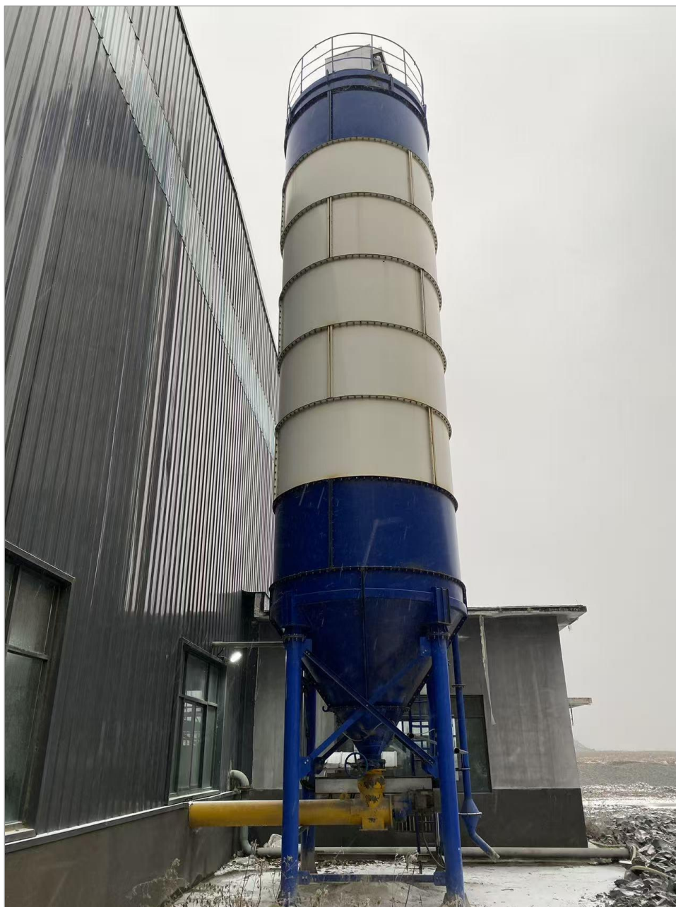
Figure 16.14 Binder silo at LMW paste backfill plant
