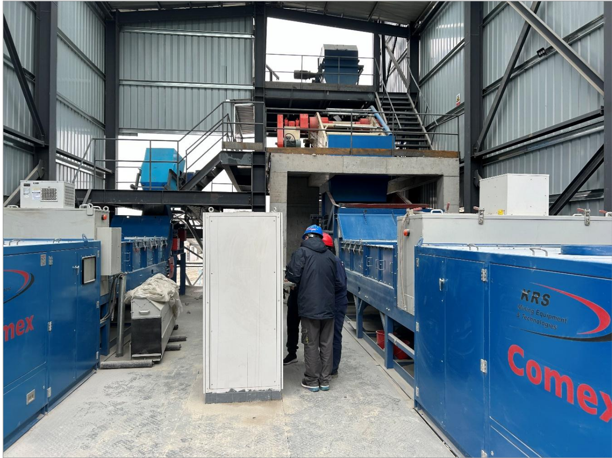
Figure 13.5 Ore sorting circuit at Plant 2 – sorting units (2)
