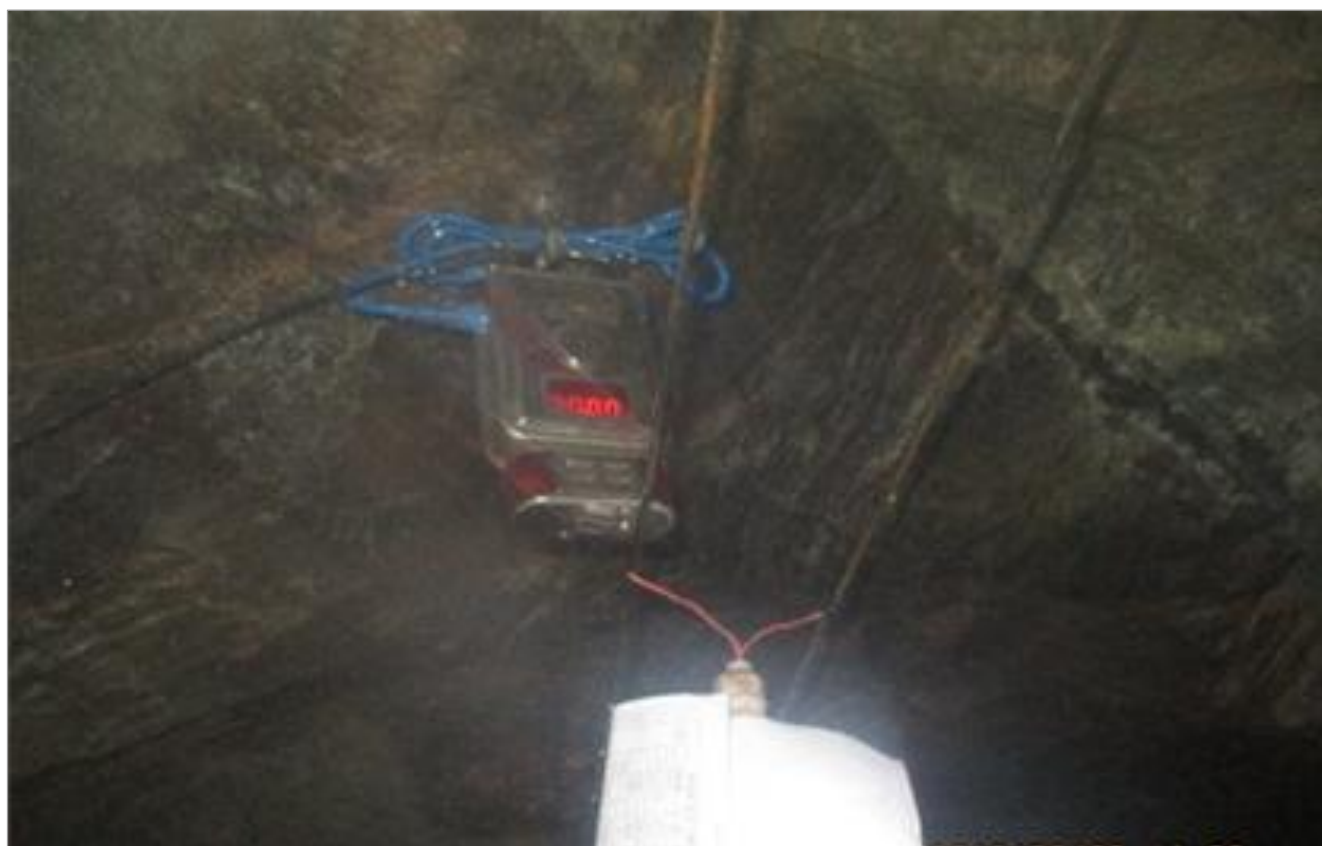
Figure 18.18 Carbon monoxide sensor at underground noxious gas monitoring system
