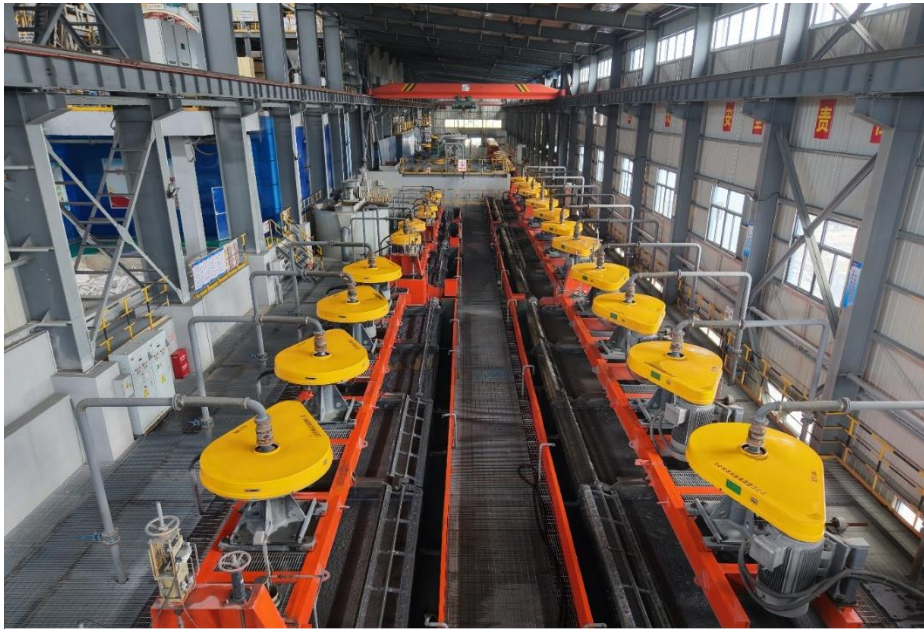
1800 TPD Flotation Line Added to Mill No. 2
