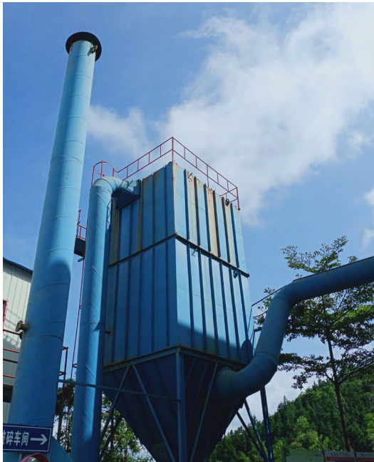
Dust collection facility
