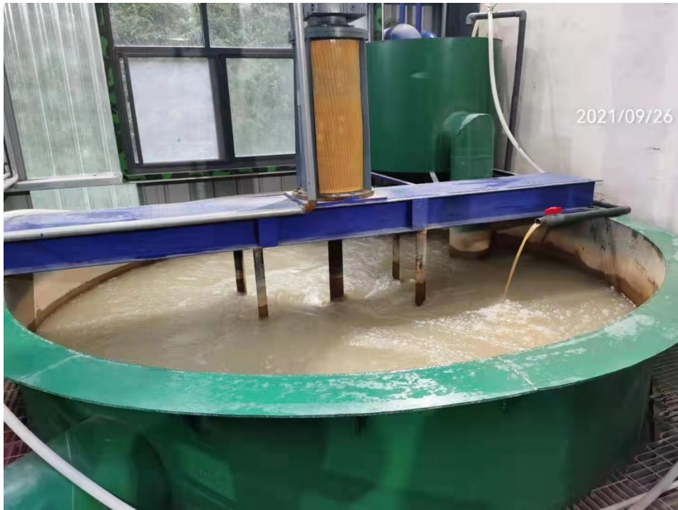
Figure 2. Mixing Tank with Reagent Addition
