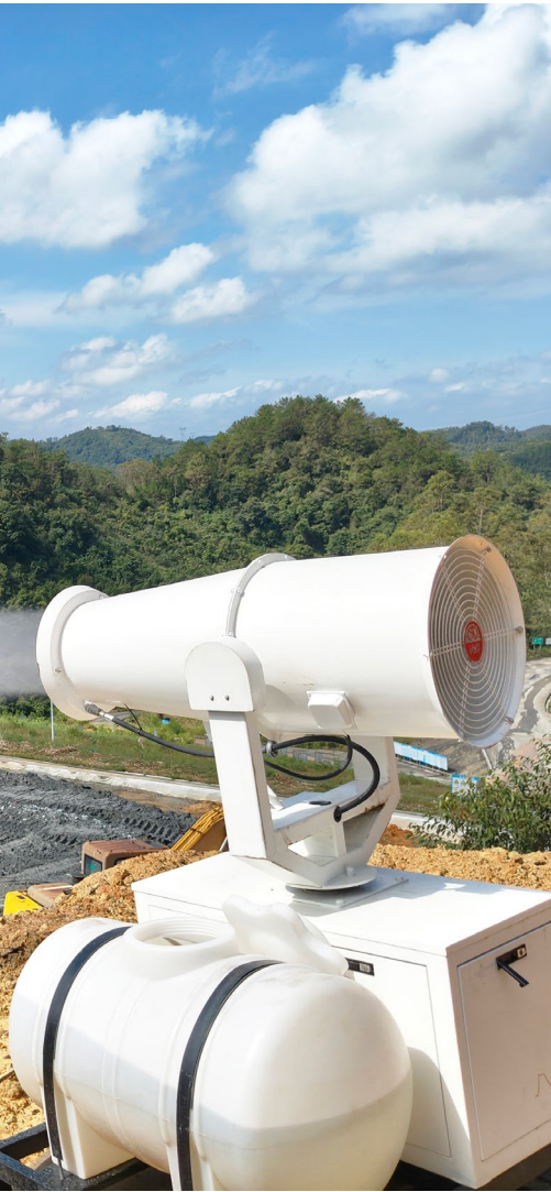
Fog cannon at the GC Mine dry-stack tailings facility, Guangdong Found
