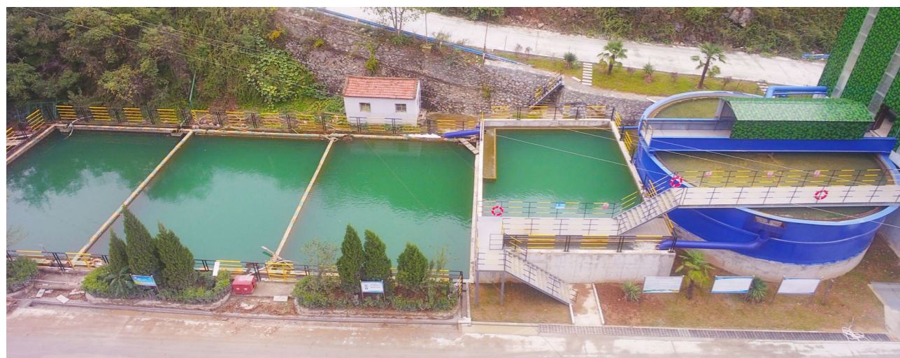
Environmental treatment facilities for gushing water in the sand ditch mines of Henan Found
